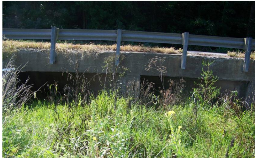
Figure 7: Sediment build up on the upstream side
